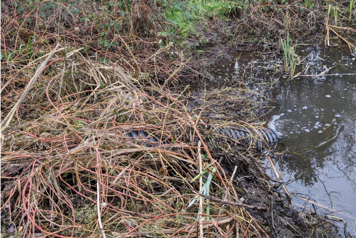
Figure 15. Pond leveler device - flexible pipe allowing water to flow through dam.
