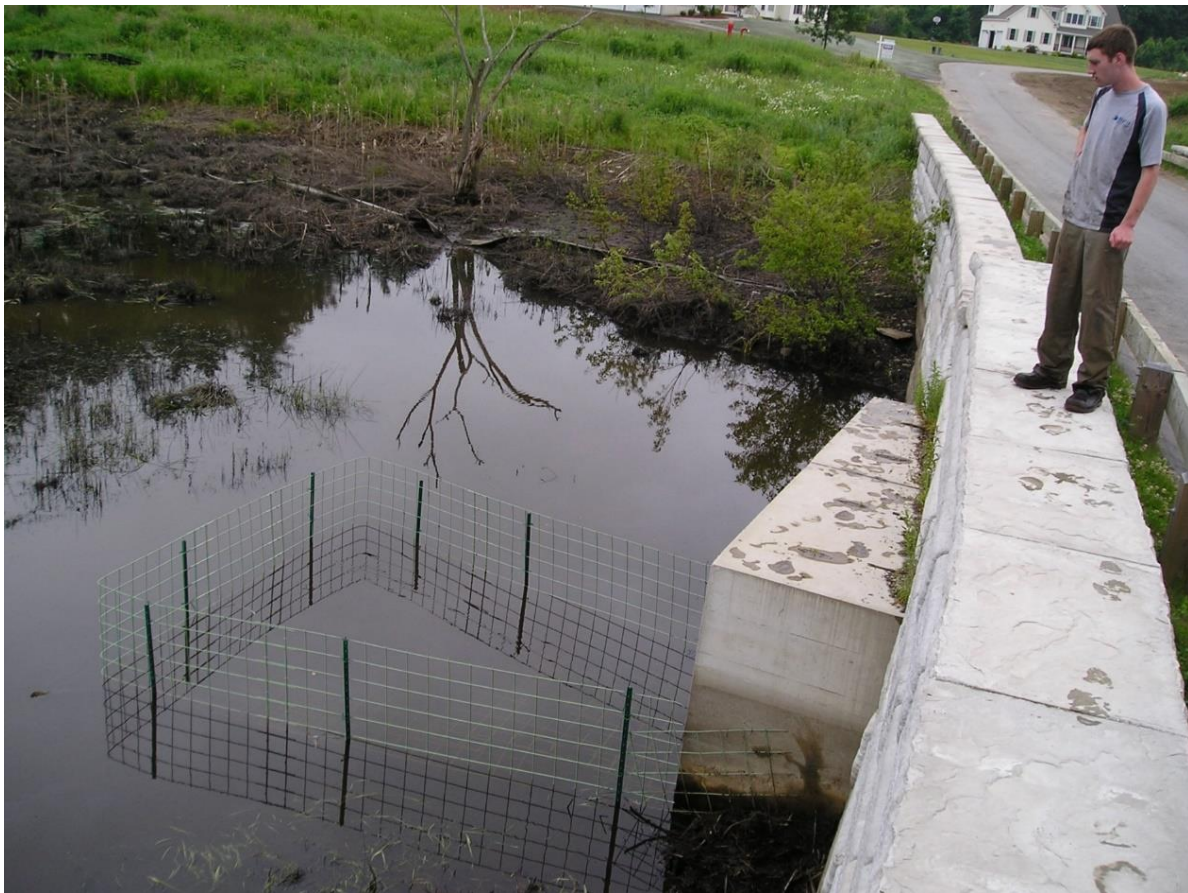
Figure 16. Trapezoidal fence to protect culvert in Massachusetts. Photo by Michael Callahan ( www.beaversolutions.com ).
