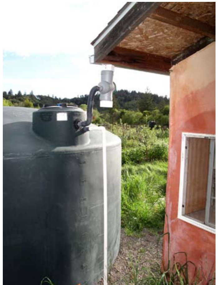
Roofwater harvesting system at Salmon Creek Middle School in Occidental, CA
