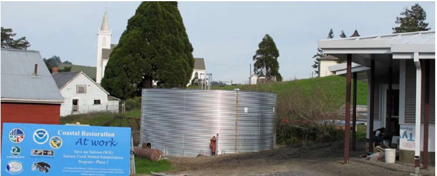
Front view of Bodega Volunteer Fire Department's new roofwater catchment system installed by the SOS program in Bodega, CA
