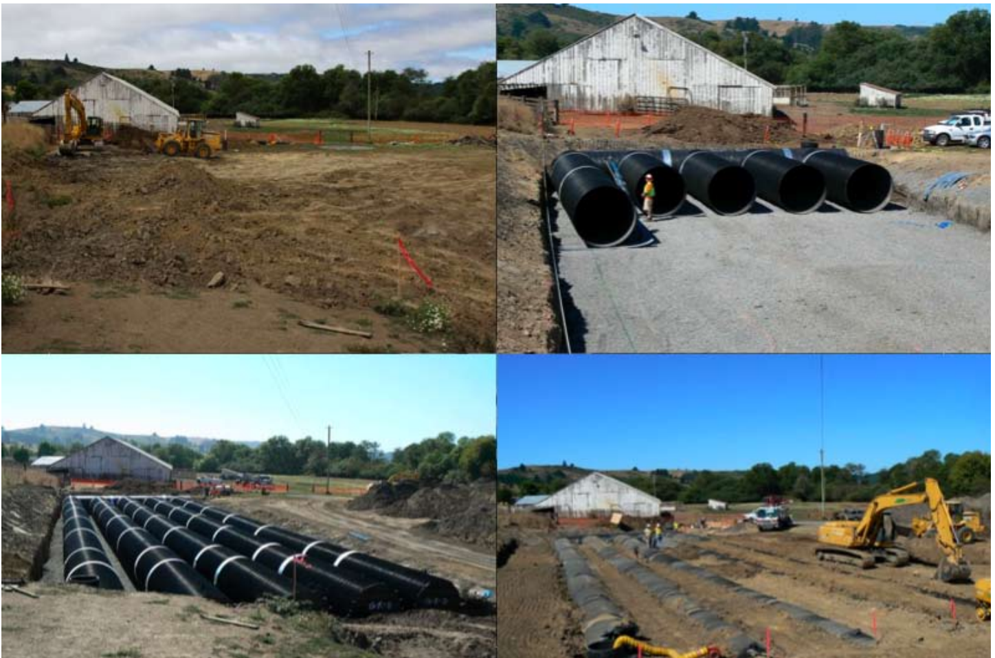
Gilardi Ranch Roofwater Tank - Gold Ridge RCD & Prunuske Chatham, INC. Photos by John Green Underground tanks store rainwater from the roof of this dairy barn. Installed by SOS program in Bodega, CA
